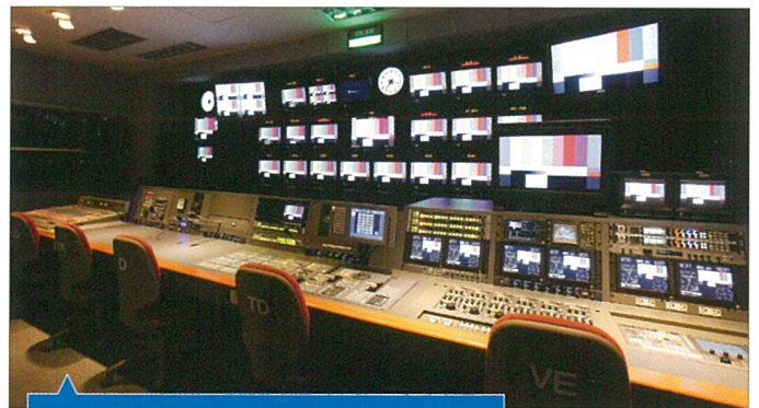
TV Studio Sub-control Room
